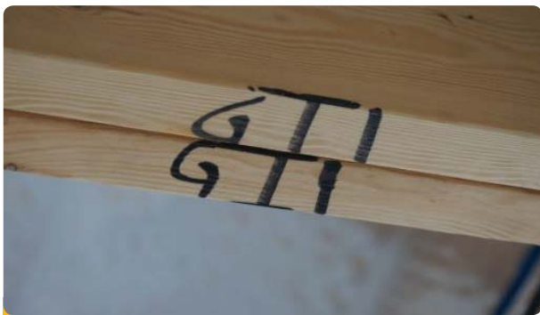
Typical placement identification marking to the underside of a bottom truss chord
