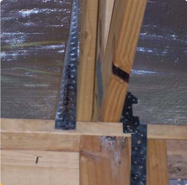
Inappropriate tie downs
