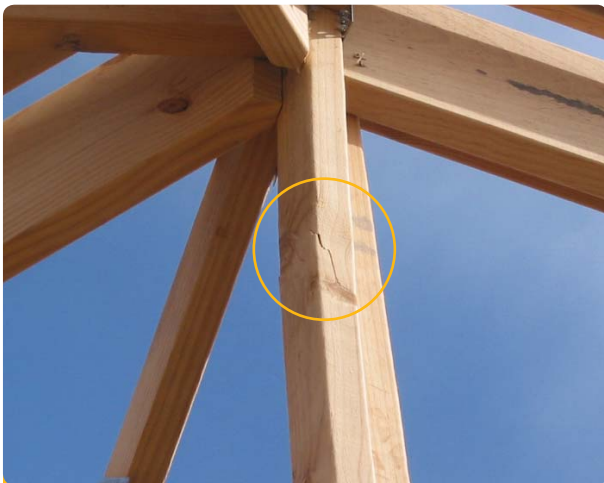
A cracked strut member supporting a roof apex joint assembly
